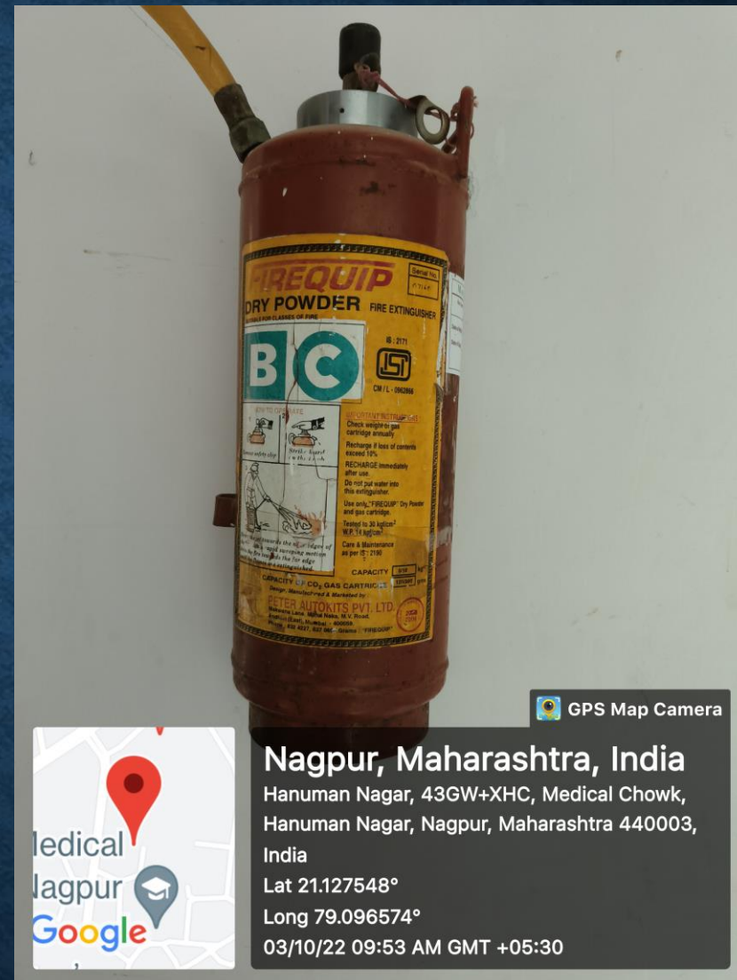
FIRE EXTINGUISHER FACILITY IN GDC, NAGPUR
